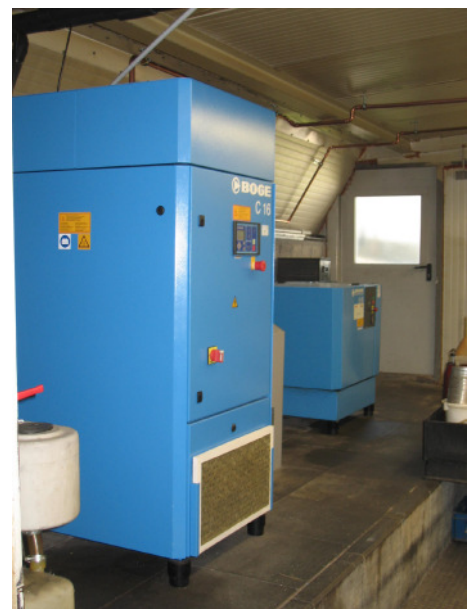
Failure safety: 2nd compressor for the compressed air supply system
